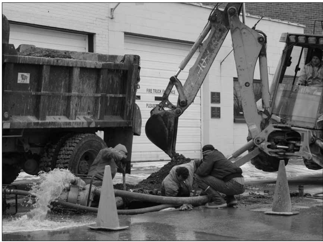
A city maintenance crew works to repair a water line on East Bellville Street Tuesday.
