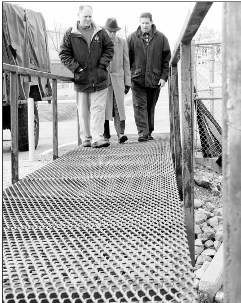
City Attorney Bart Frazer, Mayor Mickey Alexander and school Transportation Director Al Starnes take a look at the old metal bridge connecting Elm Street to the school campus.
