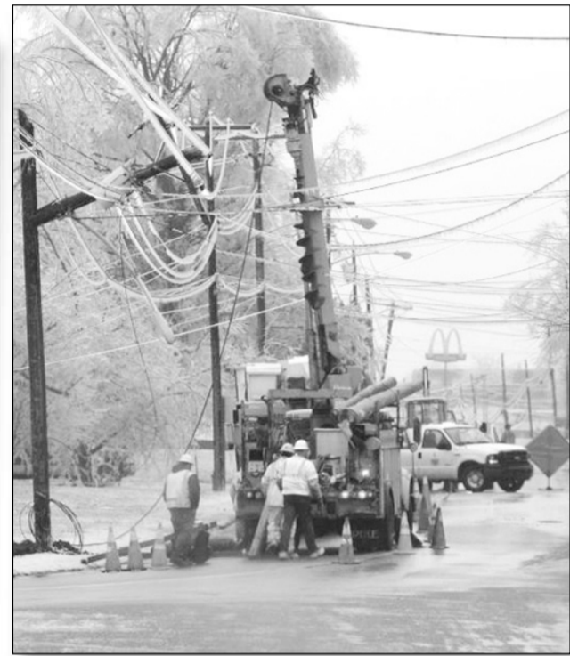
PHOTO BY JANSON JAMES Power company workers repair the broken pole on North Main Street.
