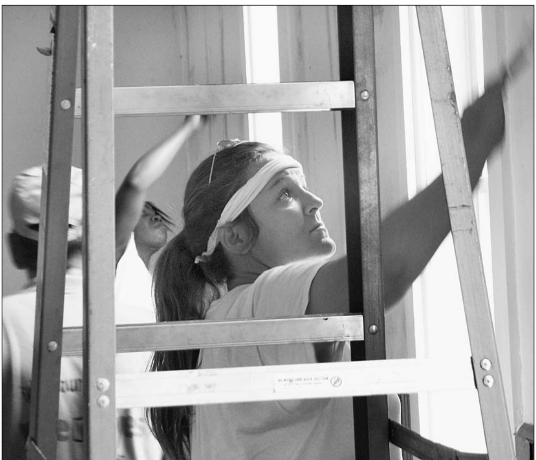
Toni Johnson (foreground) and Juanita Riley prime the trim around windows Tuesday afternoon at the former Blackford Church of God at the head of the Blackford Walking Trail and Walk of Honor. The church is being converted to a visitor's center.
