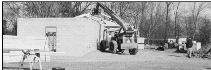
Construction sites are commonplace right now in Marion. Above is the new county animal shelter going up behind the county garage. At right is the PACS Senior Center addition.
