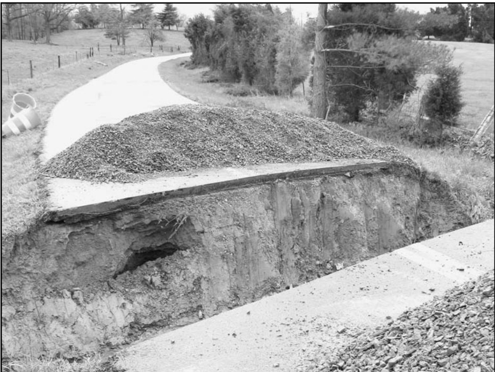
Sisco Chapel Road (Ky. 2132) near Midway remains washed out from the torrential rains that fell in Crittenden County earlier this month.
